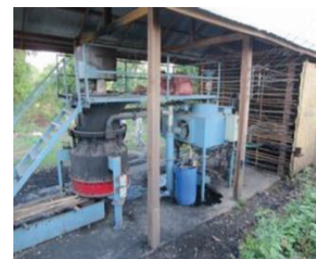
Bagasse power plant of Hoang Anh Sugar Mill was installed in Phouvong, district Attapeu Province with the capacity of 30 MW.
